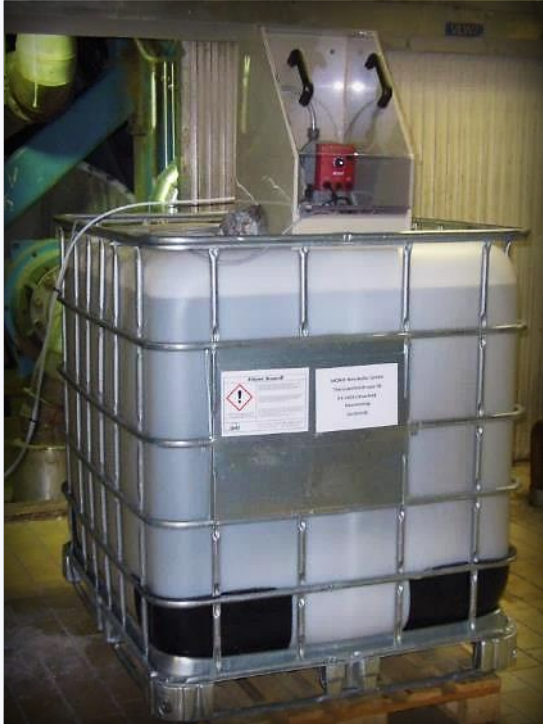
Passivation fluid tank, with dosing pump
